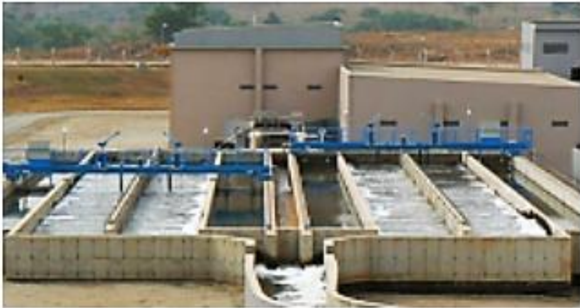
Figure 3 Shows Abuja Wastewater Treatment Plant
